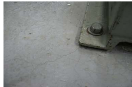
Figure 1. Crack at Control Panel
